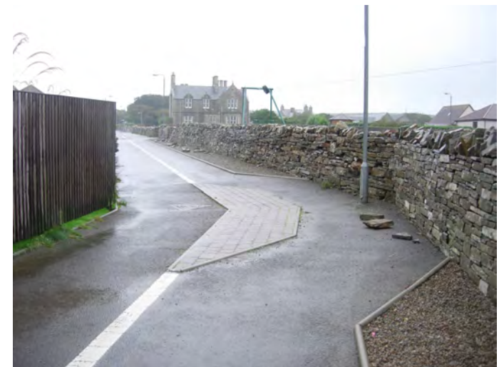
Dividing strip 'forces' cyclists to cycle towards wall. Note falling masonry requiring maintenance
