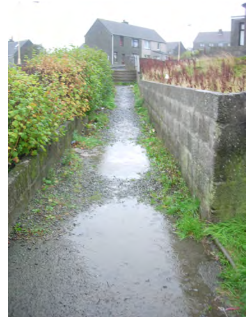
Shortcut in Quoybanks requires surfacing and steps replaced with DDA compliant ramp
