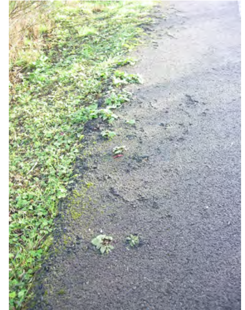
Damage to Weyland cycle track from invasive weeds
