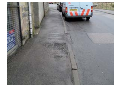
2E - Damaged and uneven footways along Roding have caused drainage issues
