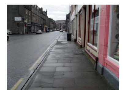
2B - Uneven block paving along Long Row could cause trip hazard for pedestrians
