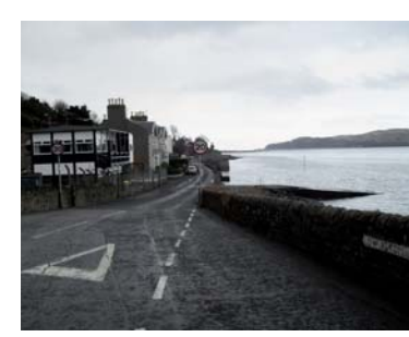
1B - No provision for pedestrians exists along Low Askomil Walk which leads to conflict with vehicles and other road users
