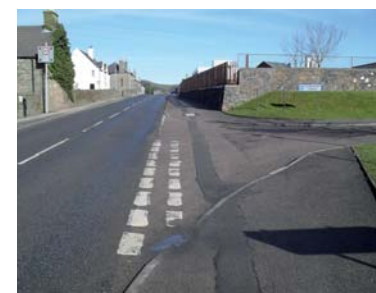
4C - Drainage is an issue at Campbeltown Hospital entrance as is the wide mouth on the junction
