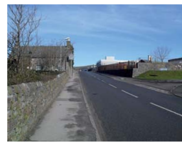
4B - Narrow footway on Ralston Road presents conflict point for pedestrians
