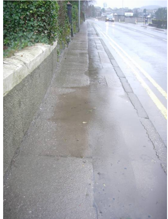
Figure 5.12: Ponding on Argyll Road
