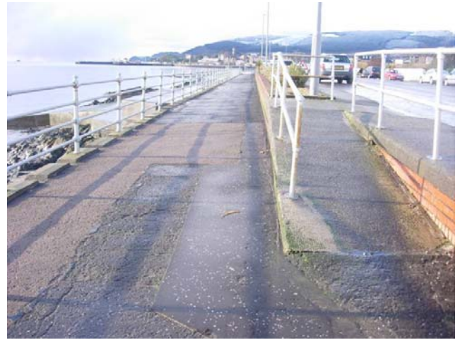
Figure 5.19: Surface deficiencies on promenade
