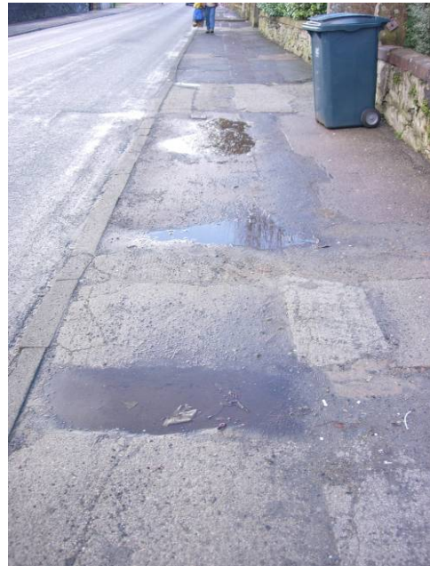
Figure 3.4: Example of ponding on footway
