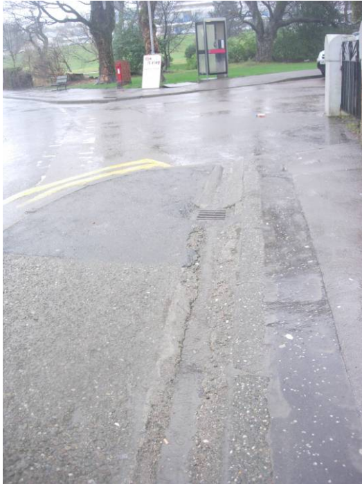
Figure 5.11: Poor quality footway on Sandbank Road
