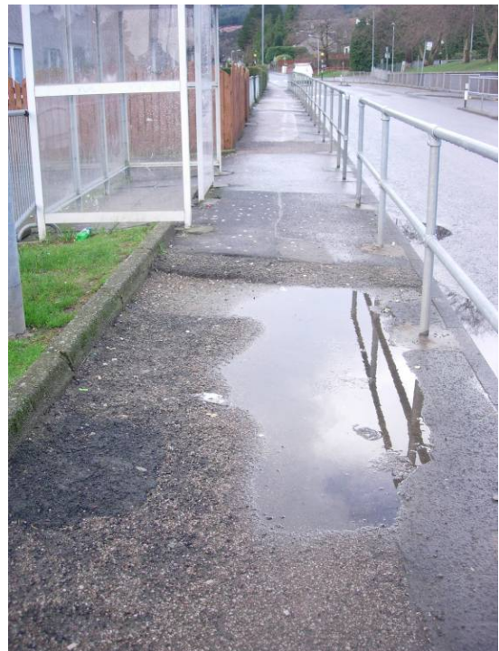
Figure 3.6: Example of ponding on footway
