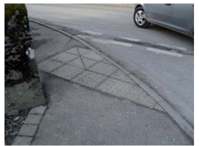
2B - Tactile paving randomly placed and is poorly maintained
