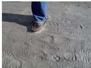
1C - Poor surfacing on NCN 78 retains water
