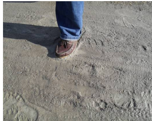
Figure 3.4 – Poor surfacing material – NCR78
