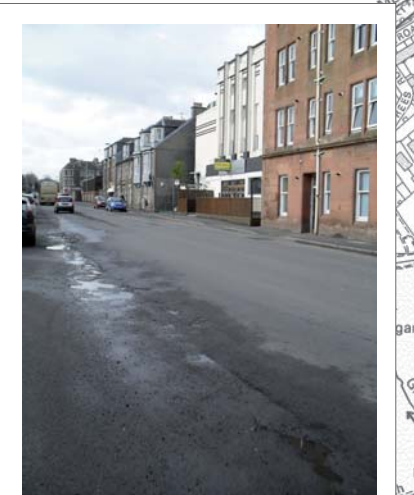
2H - Surface quality is poor with accompanying drainage issues
