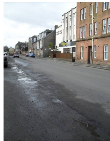
Figure 3.3 Inadequate surfacing on High Street
