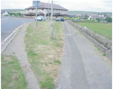
4a The pedestrian facilities at the junction of the A9 and A836 do not serve pedestrian desire lines.
