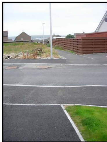
Figure 3.34: Poor continuity between pedestrian paths in new development
