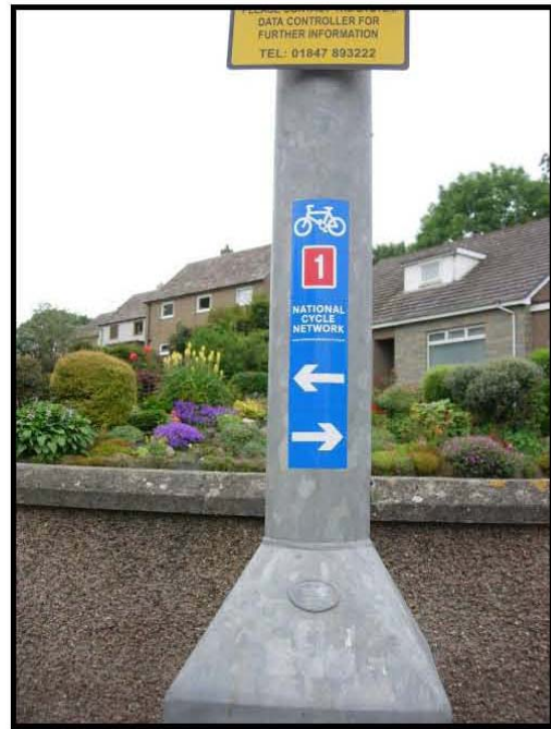
Figure 3.27: Poor quality signing on Route 1
