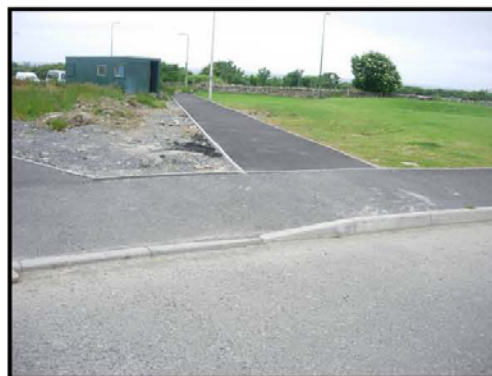
Figure 3.36: Dropped crossing does not serve pedestrian path in new development
