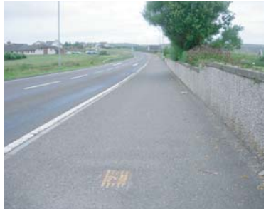
4a The footway on Scrabster Road could be easily converted to shared use for cyclists and pedestrians.
