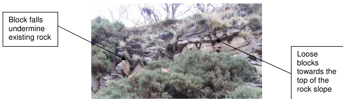
Photo 7.1 Weathered rock and loose rock blocks on roadside rock cut
