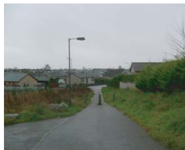
4k The road closure at Old Miniarfua Road / Obsdale Road is becoming overgrown.
