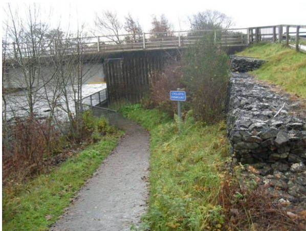
Figure 5-7: Sign instructing cyclists to dismount due to low overhead clearance and poor sightlines at underpass of A9.
