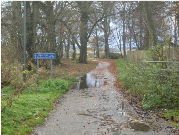
Figure 5-5: Signage for Alness Point Business Park at Riverside Drive to the south of Teaninich Industrial Estate. Note poor drainage along route and maintenance required to clear leaves and debris from path
