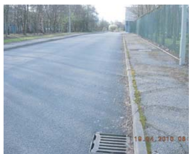
6h Existing footways are in poor condition in Inverbreakie Industrial Estate.
