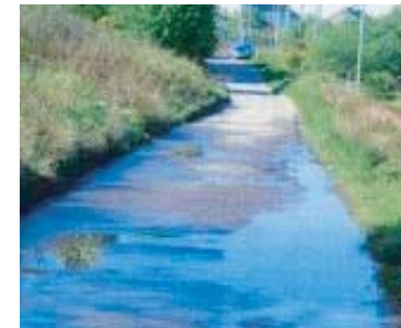
1e A section of road through Black Park is often wet. Improved drainage would help to make the route more attractive.
