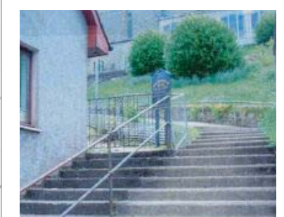
6c The steps provide a good short cut to the town centre. However there is evidence of drinking and urination.
