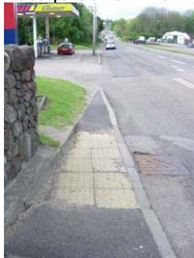
Figure 3-8: Poor quality footway provision on A82
