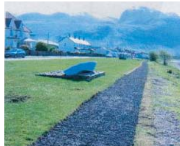
A new footway is under construction in Caol, although it is not of sufficient width to allow shared use between pedestrians and cyclists. This area has flooded in the past and is under a Flood Prevention Order.
