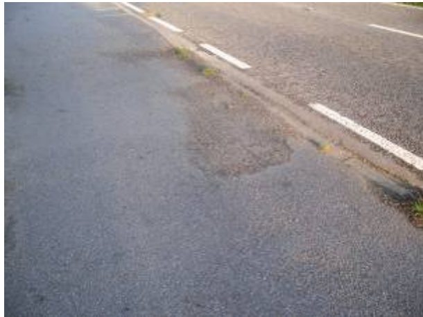
Figure 5-61: Debris and gravel accumulates and causes puncture hazards
