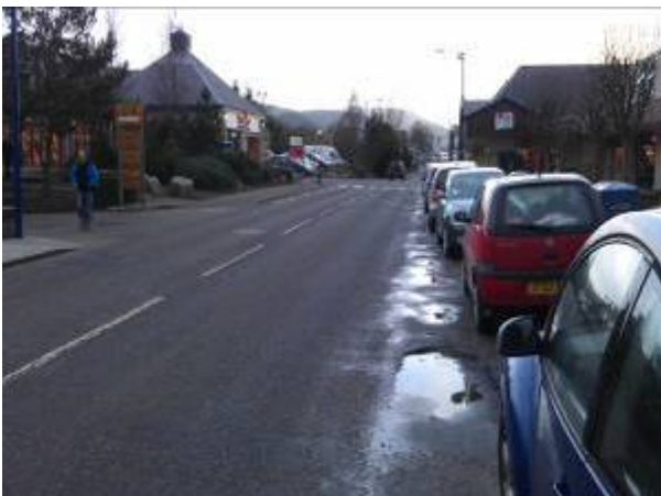
Figure 3-5: On street parking, poor surface condition and Zebra crossing next to Tesco
