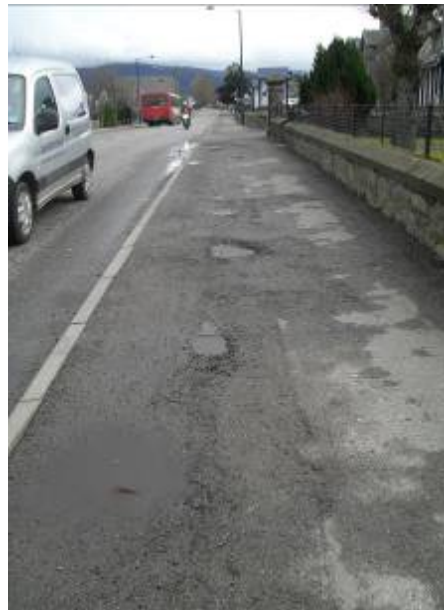
Figure 5-4: Poor footway maintenance symptomatic of Grampian Road
