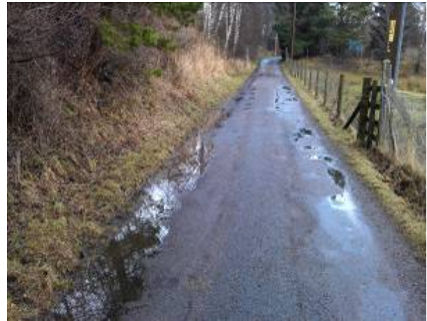
Figure 3-16: Traffic free NCN route running parallel with Grampian Road showing poor surface drainage
