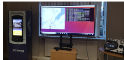
Automated train describer equipment
